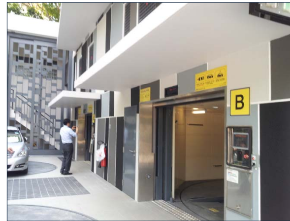
Dual Turn Table at internal and external .
